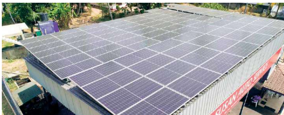
Green Atom company Pvt Ltd., Solar project which funded under ADB rooftop solar loan scheme.
